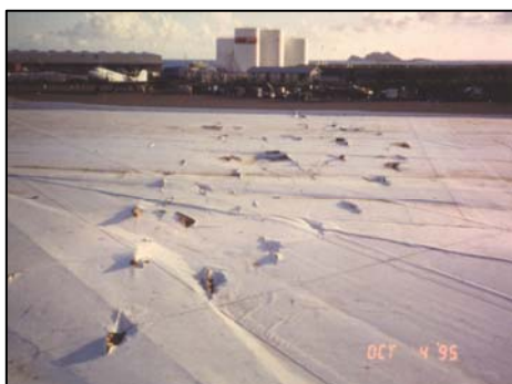
Figure 2. Roof cover damage from equipment Source – FEMA=
