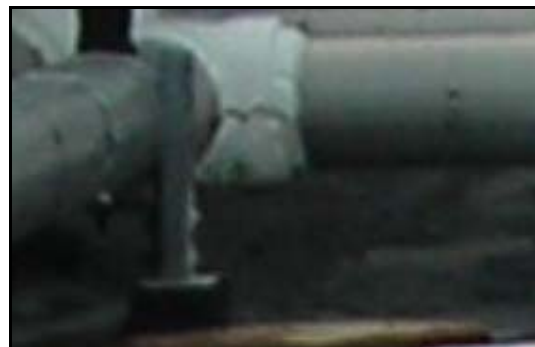
Pipe supported on stands anchored to concrete deck
