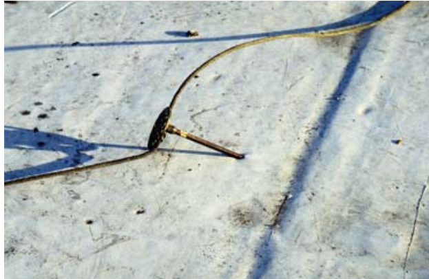
Air terminal penetrating roof cover (source FEMA)
