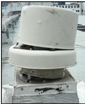
Wind damaged fan and cowling
