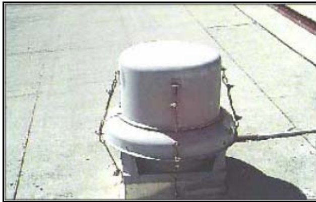
Secured fan and cowling Source - FEMA
