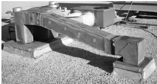
Exposed rooftop ductwork
