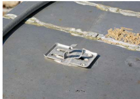
Conductor separated from clip after high wind Source – FEMA
