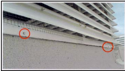
Inadequate securement Source – FEMA
