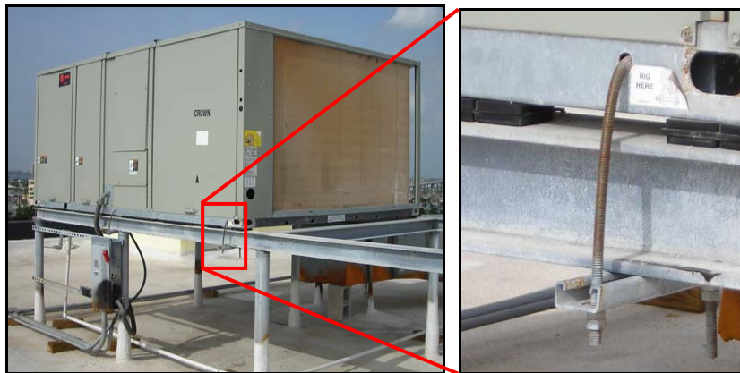
Example of a non-engineered connection anticipated to fail under high winds
