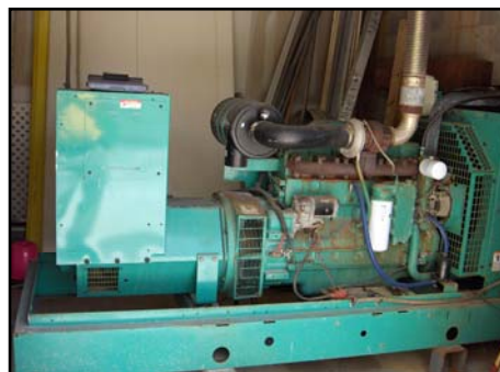
Figure 1. Diesel engine driven emergency generator
