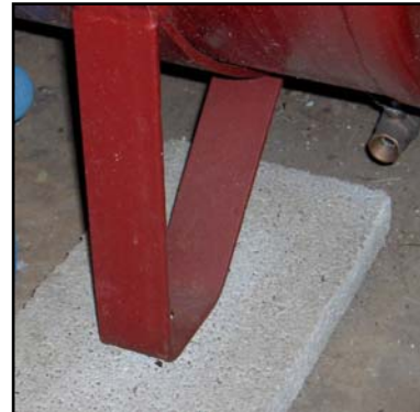
Figure 5. Fuel tank leg not bolted to floor
