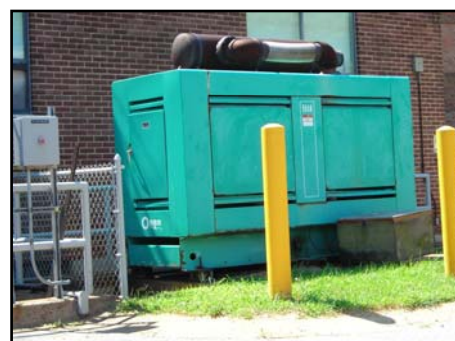
Figure 2. Bollards provided to protect emergency generator from physical injury
