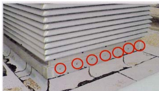
Adequate securement (Photo source – FEMA)
