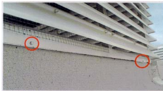
Inadequate securement (Photo source – FEMA)
